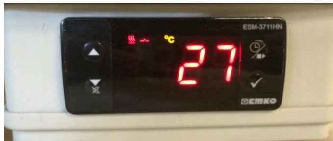
Figure 4. Temperature controller switched on
