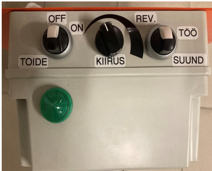
Control panel of the pump
